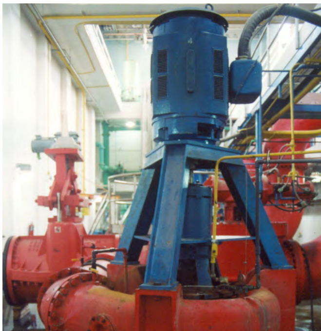
Pumps that are wasting energy often look and sound just like other pumps in the system. The only reliable way to ensure efficiency is to use calculations, field measurements, analyses, and data. Tom Walski
