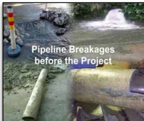
Pipe breakages before the project
