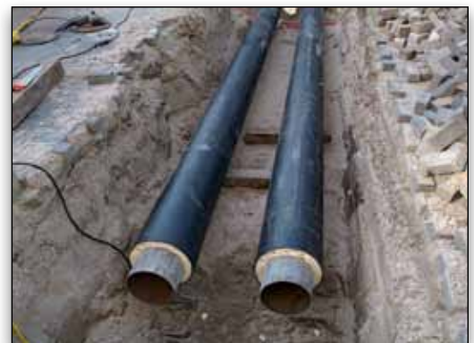
Bentley sisNET is used to support the operations phase of the lifecycle for ELES's district heating network.
