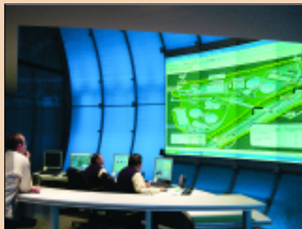
Typical SCADA control center
