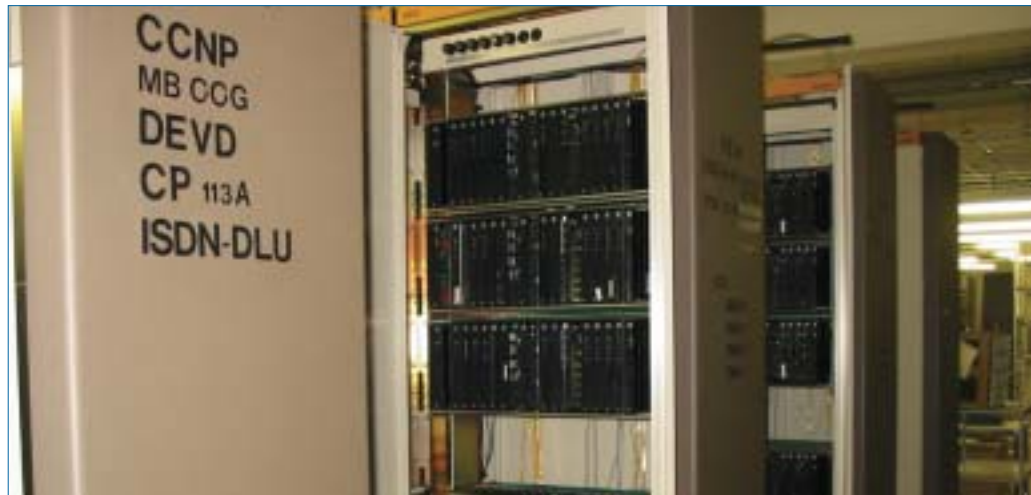
The Document and Premises Management System handles information about 310 central offices and 9,500 racks.
