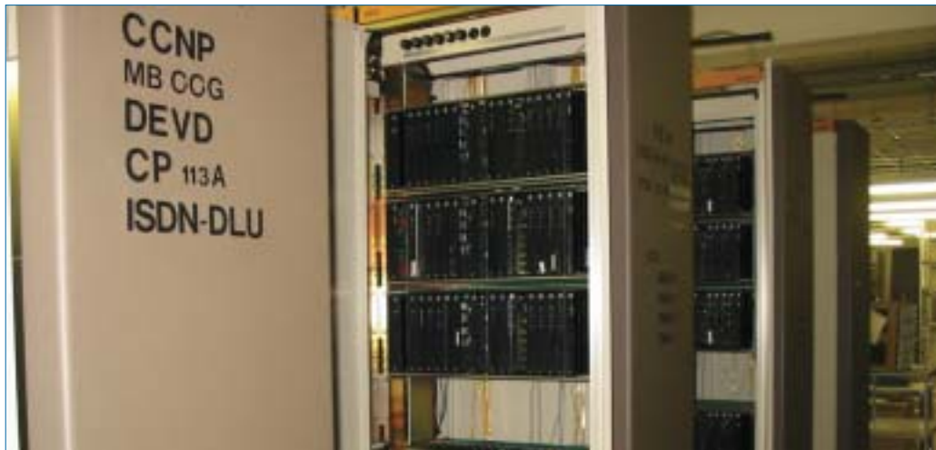
The Document and Premises Management System handles information about 310 central offices and 9,500 racks.
